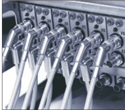
Figure 4 . 90-degree and 45-degree angled connectors help route cables away from the box in an orderly manner.
